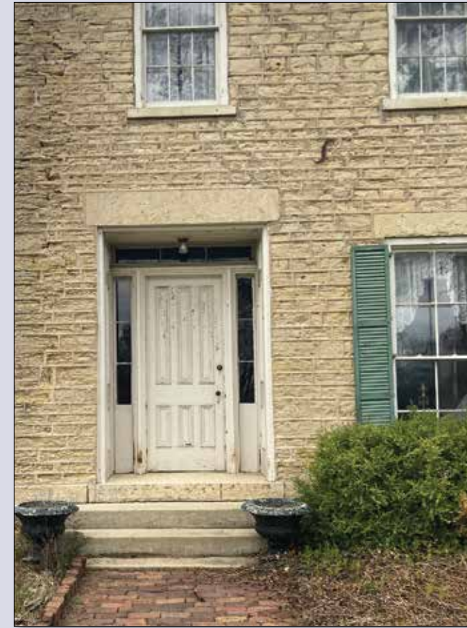
Hanchett-Bartlett Homestead view of front entrance looking north showing four uneven risers and a brick path that has settled. April 13, 2022
